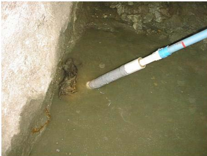
Figure 4: Monitoring ANZI strain cell about to be installed 40m into a BQ borehole.
