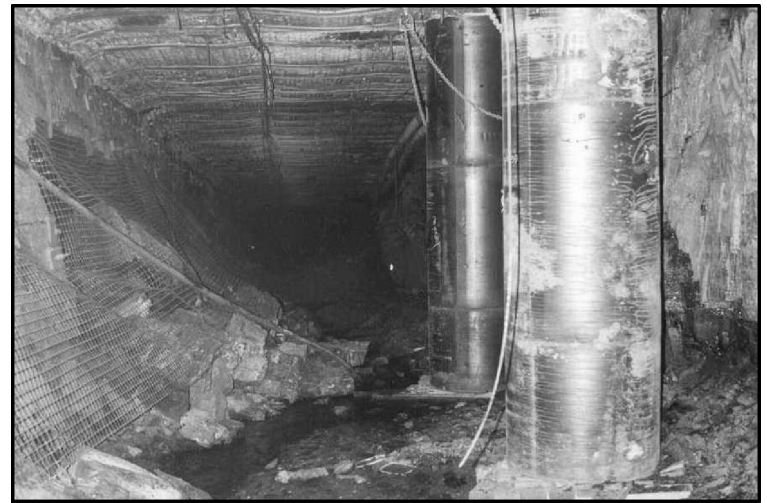
Figure 5(d) Rib deterioration threatens serviceability of roadway as a travel road above 15MPa vertical stress.
