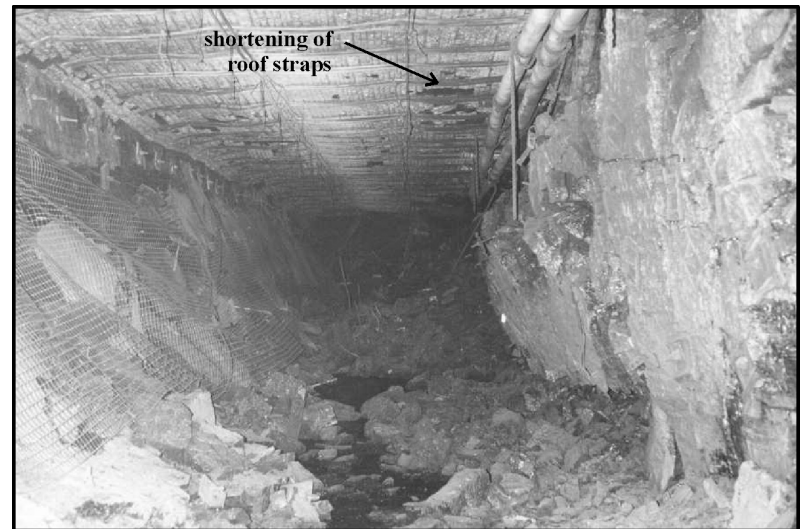
Figure 5(e) Roadway conditions are severe and potential for roof falls becomes an issue above 20MPa vertical stress.
