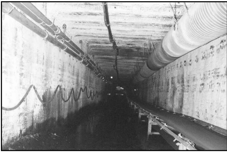
Figure 5(a) Excellent roadway conditions when major stress is vertical and less than 6-7MPa.
